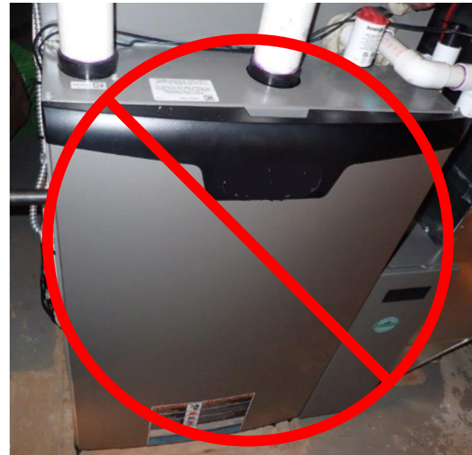
New Condensing Furnace
