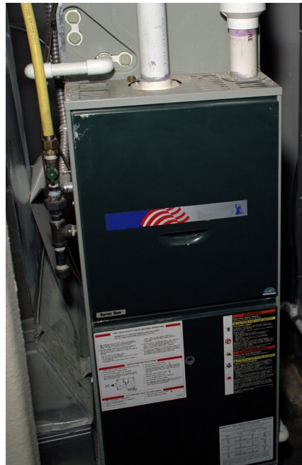
Existing Condensing Furnace
